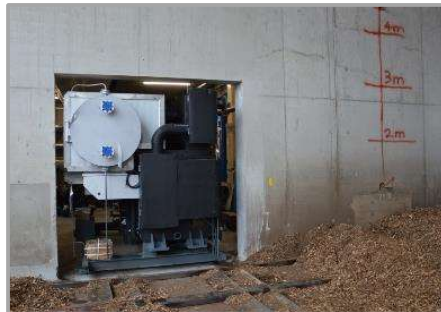
Strass, 2021 Heat recovery 500 kW
